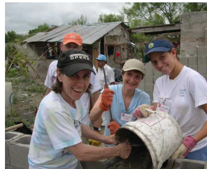
From left, Dave Johnson, Jennie Betton, Diane Bishop, and Emily Hoxworth pour concrete during the July 2006 Mexico Mission trip.
